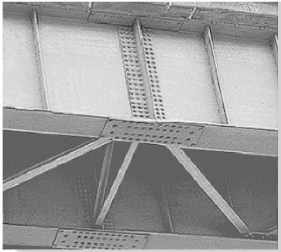
Shown are typical splice plate joints used to connect the steel girders of a highway bridge.
